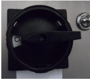
Figure 2. Main switch "off"
